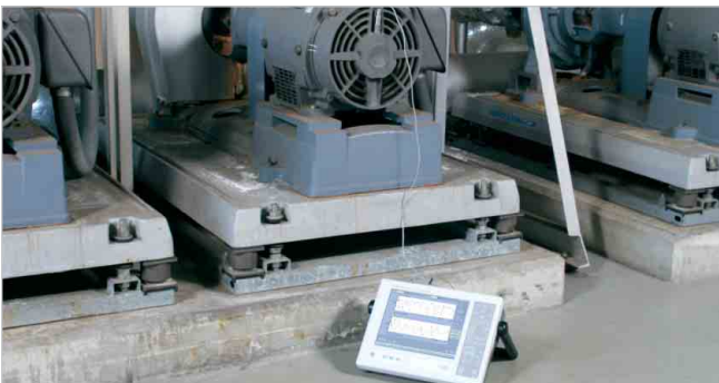
Vibration measurement in a plant using the CF-7200 and an NP Series Acceleration pickup
